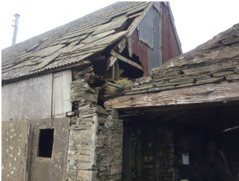
Photo 9. Hopefield barn - corner of barn with large access area into the barn
