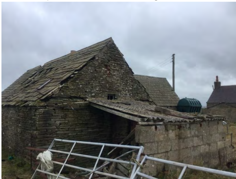
Photo 10. Hopefield stone barn with missing tiles
